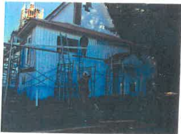
Priest's Quarters: Gutters, reconfiguration of a door to a window (left) + new door facing front of the church (Photo: Robin Inglis, Fall, 2017)
